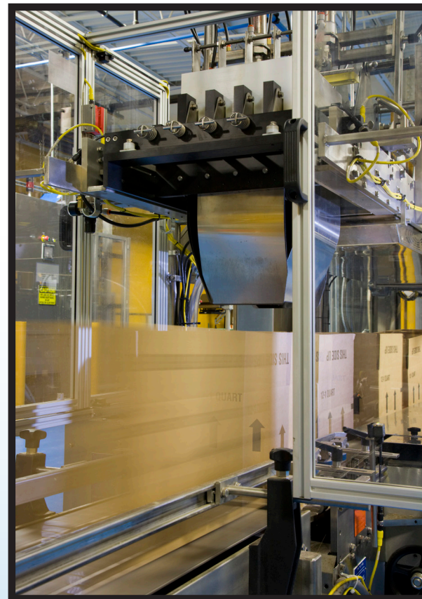
A packaging machine using T-slotted aluminum rail as an enclosure around the working parts of the machinery
