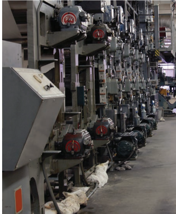
Figure 3: Web printing presses, paper mills, and material converting applications require the precise speed regulation of closed-loop control available in higher-end VFDs. Elsewhere, volts-per-Hertz (V/Hz) and sensorless (or open-loop vector) modes are used.
