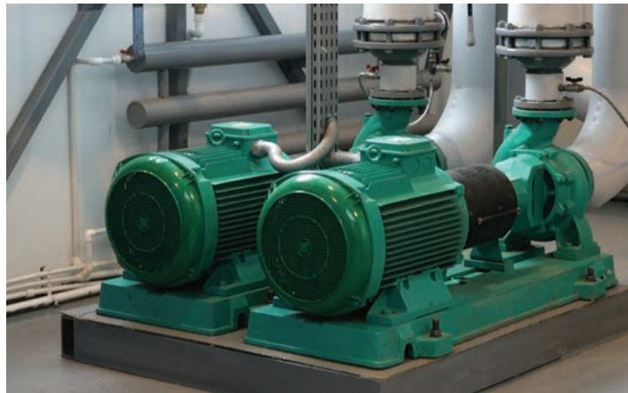
Figure 2: Using VFDs to operate fans and pumps can significantly reduce energy consumption, because they can tailor fan speed to the application. Fan horsepower is proportional to the cube of fan speed, so depending on motor size, energy savings can compensate for the initial VFD purchase price in less than two years.
