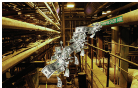
Figure 3: The average plant loses as much as 35 percent of compressed air due to leakage.
