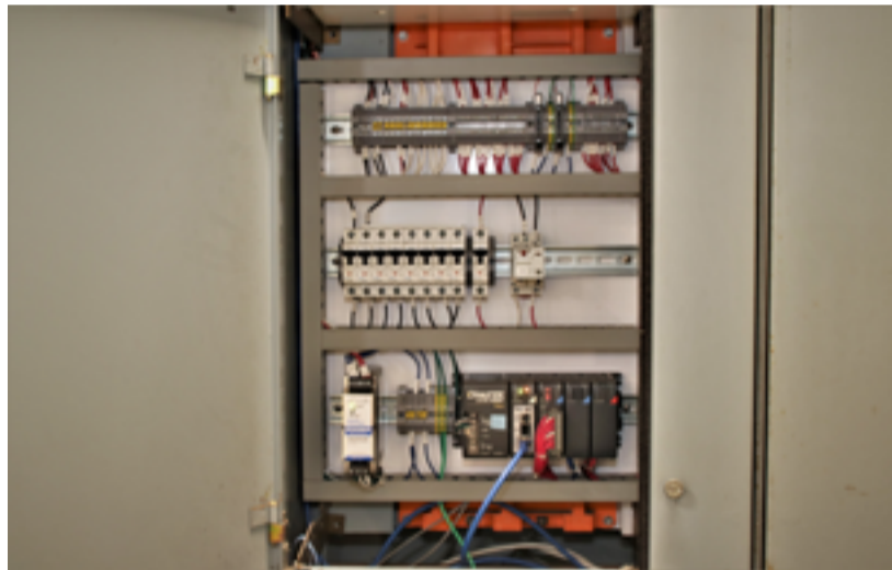
Figure 2: Inside a typical retrofitted PLC panel. Retrofitting standardized PLC panels into MCCs allows Helix technicians to more easily troubleshoot and maintain their control systems, as well as stock fewer parts while remaining ready to deal with any issues.
