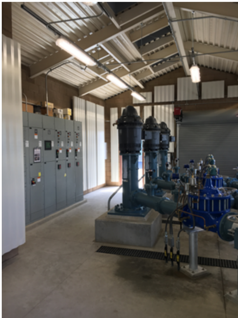
Figure 1: Inside a typical pump station. Helix Water District realized many benefits by standardizing on Automation-Direct products and best programming practices for this new pump station, and they then applied similar concepts to retrofitted stations.
