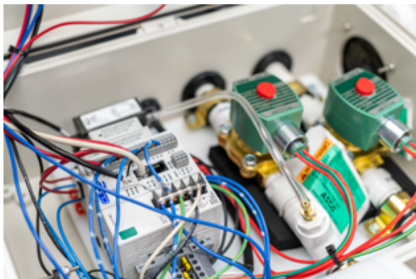
Figure 2: The readily available and economical AutomationDirect CLICK PLC made it easy to develop the ventilator, and delivered the reliability needed for such an application.
