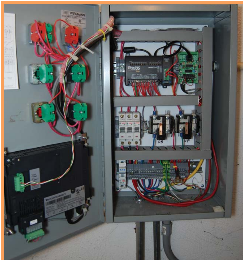
Figure 2: Micro hydroelectric plant control cabinet utilizing AutomationDirect components including a C-more Operator Interface Panel and a DL05 Micro brick PLC.
