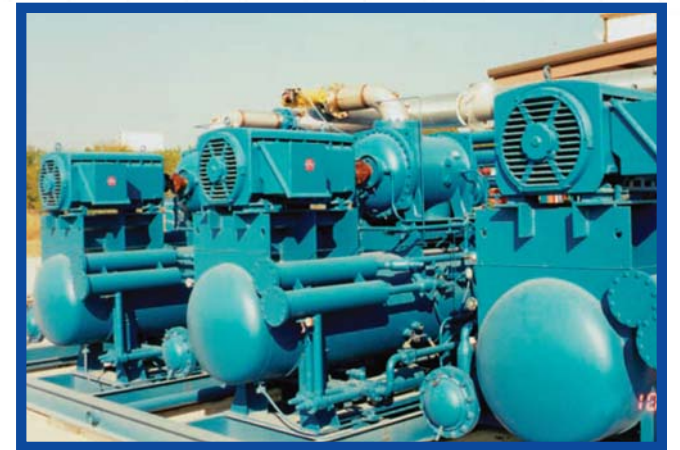
These motors are driving natural gas compressors used to compress gas from a pipeline prior to injection into a peak power gas turbine power station in Montreal. Photo courtesy of: Emerson Motor Co., reprint with permission from Plant Engineering
