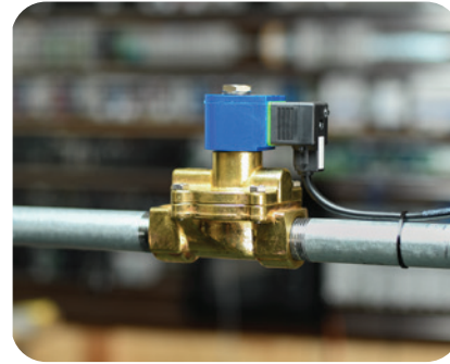
Installed process valve
