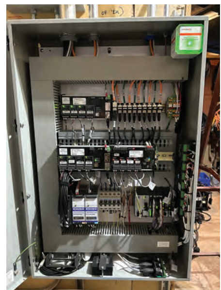
● Figure 2: The versatile AutomationDirect BRX PLC takes center stage in the upgraded house/work lighting control panel, interfacing with all other HMIs, remotely located pushbuttons, and lighting elements via Ethernet, discrete I/O, and/or DMX serial communications. All figures courtesy of Ryan Poethke
