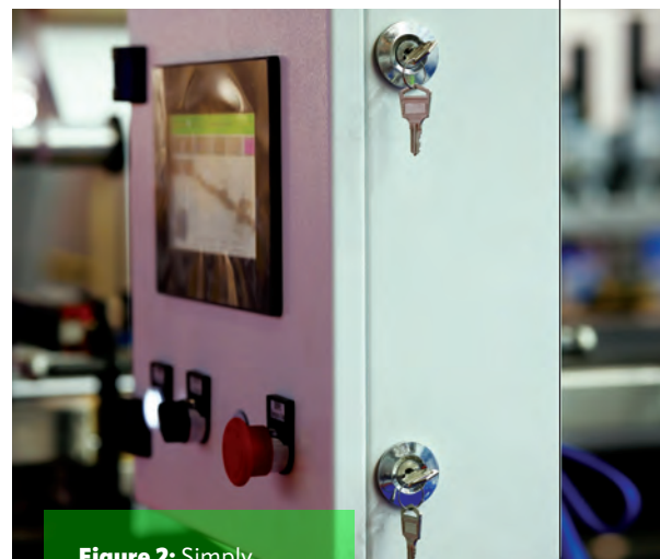
Figure 2: Simply locking up automation assets—whether in control panels, network cabinets, electrical rooms, or elsewhere—is a straightforward yet important first step toward cybersecurity.
