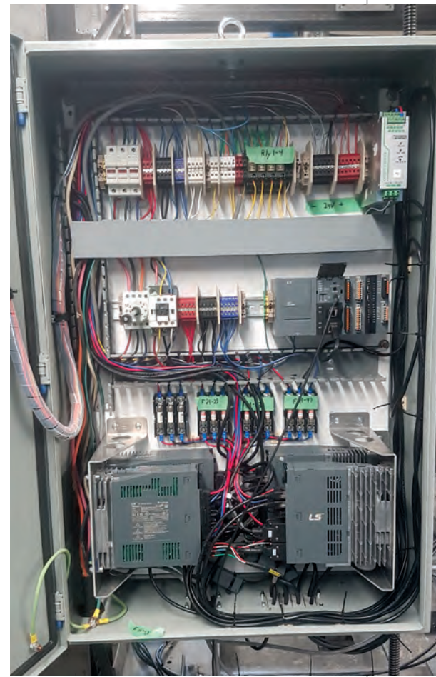
● Figure 2: The LS Electric motion controller and motor drives from AutomationDirect are shown in the team's control panel.
